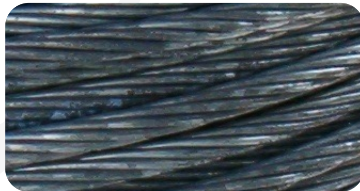
Figure 20: Oxidation on a conductor.
