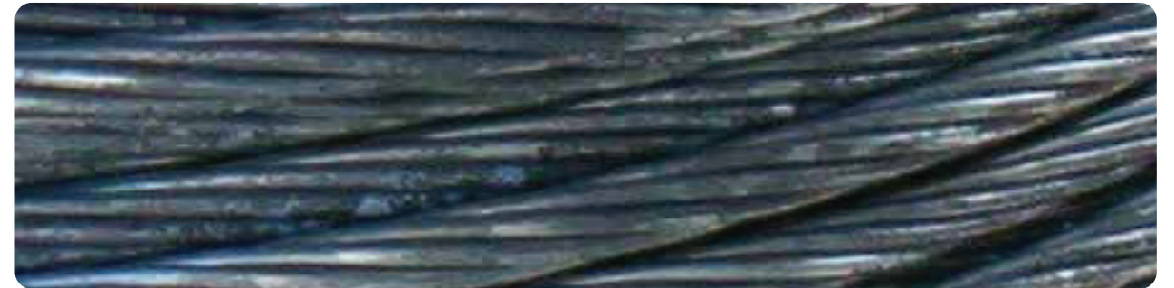
Figure 16: Oxidation on a conductor.
