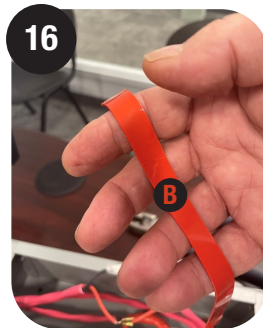
Be sure to hold onto the tape A unsecured end as you begin to apply tape B (Silicone Rubber Tape) in the reverse direction over the splice with 50% overlap as well
